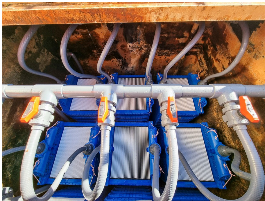
Image of Cerafiltec membranes installation for the upgrade at an existing waste-water treatment facility.
