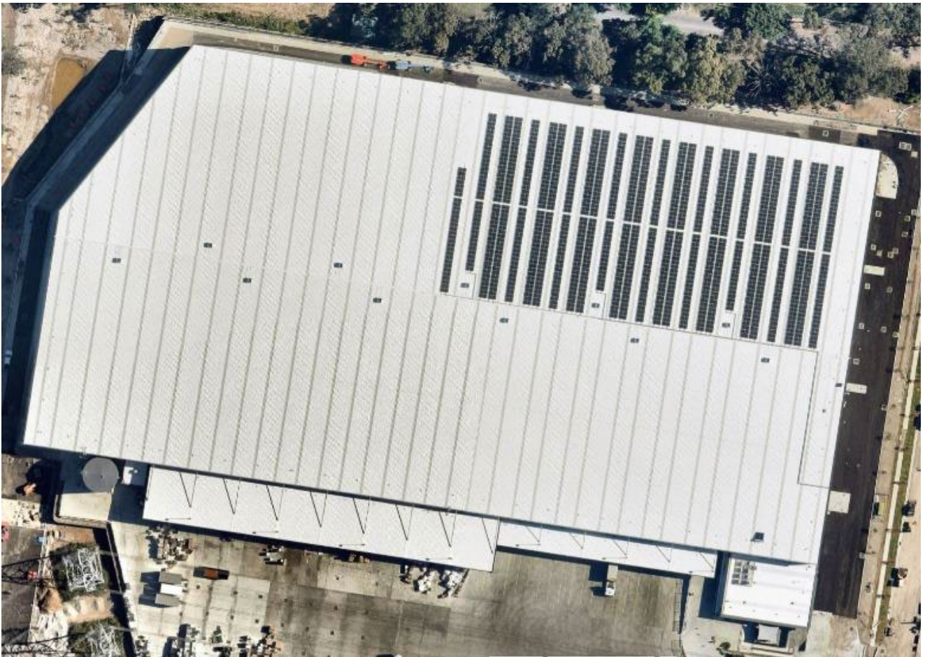
Rooftop solar panels installed at Charter Hall asset (East Logistics Park, Queensland, Australia)
